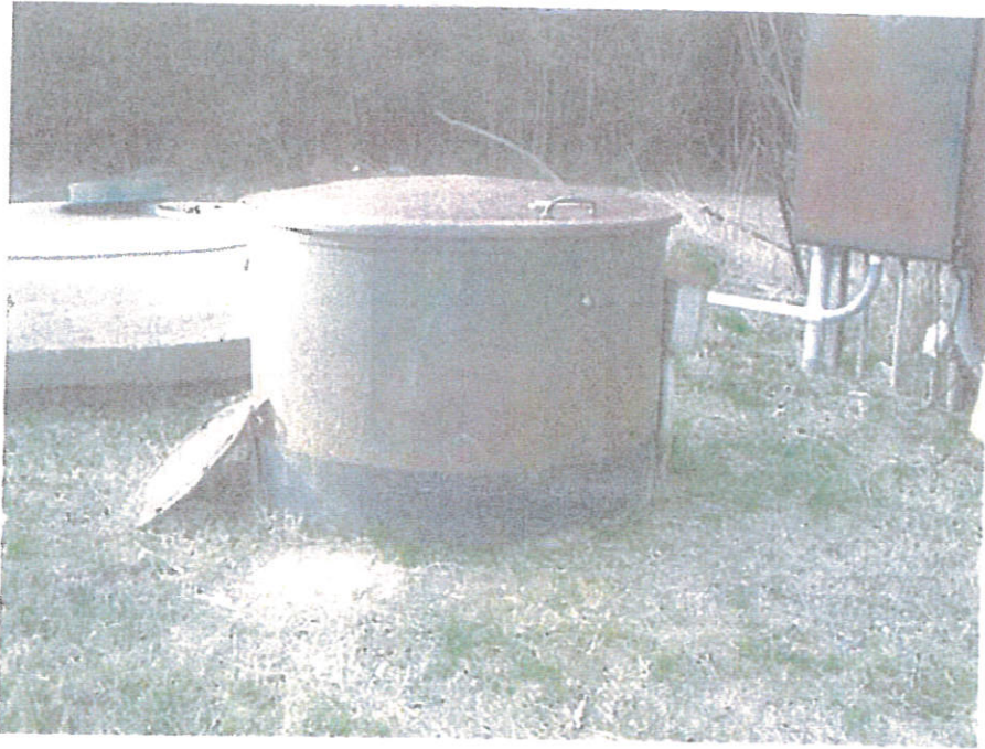
Louisville East; lift station at lagoon, Can Tex design
