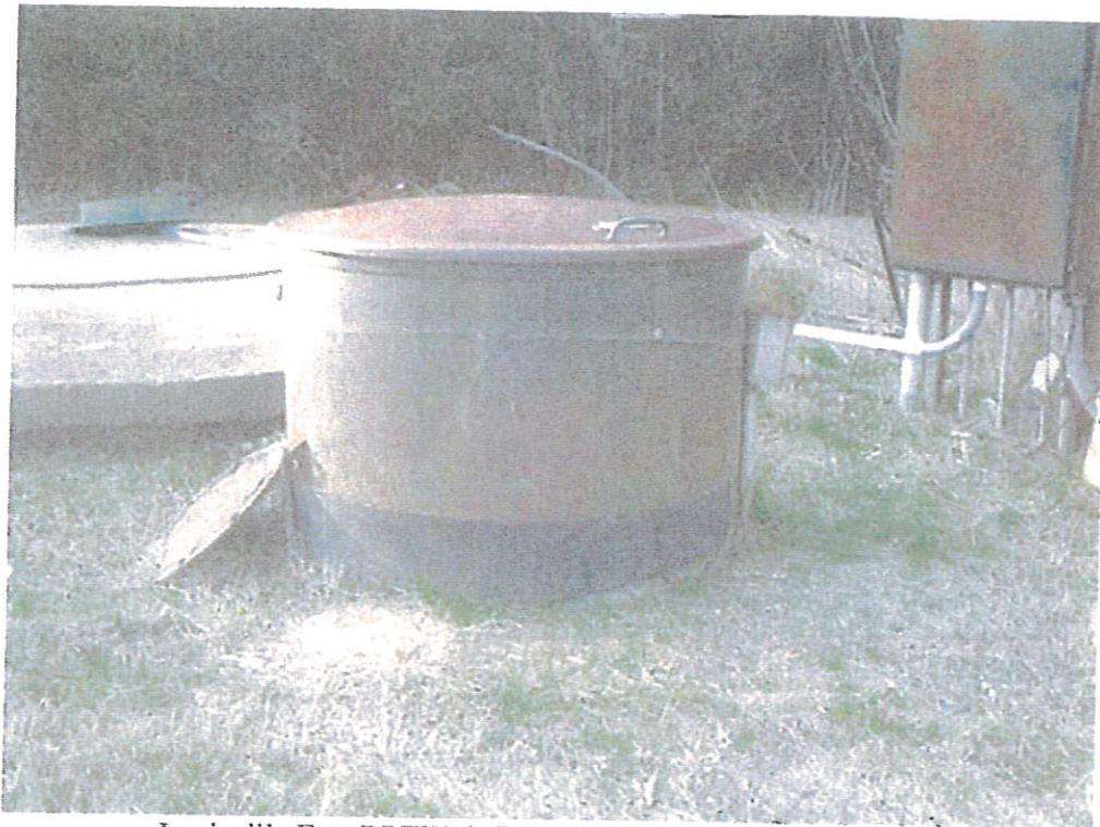
Louisville East POTW; influent lift station, 'Can Tex' design
