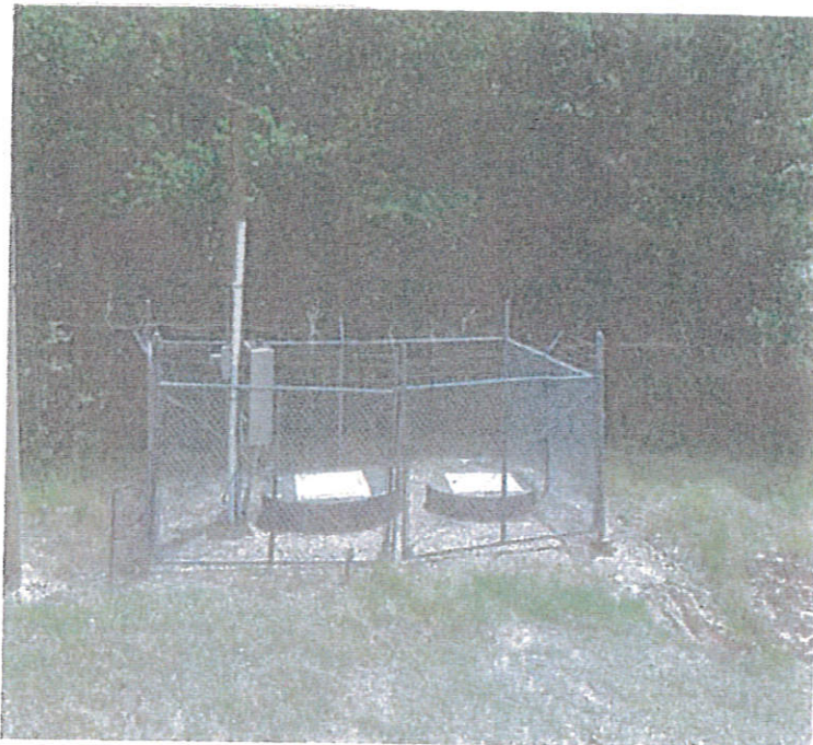
Louisville East; N. Miller Avenue lift station
