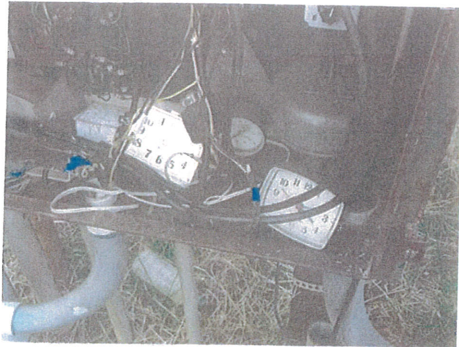
Louisville East POTW; main lagoon lift station control panel w/clocks as timers
