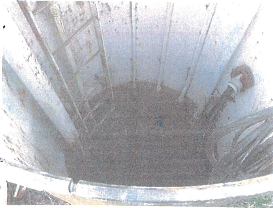
Louisville East POTW; lift station dry well ~8' depth
