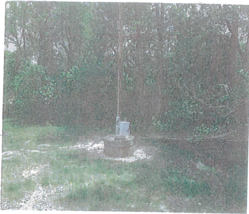
Louisville East; Johnson Street lift station, not secured/fenced
